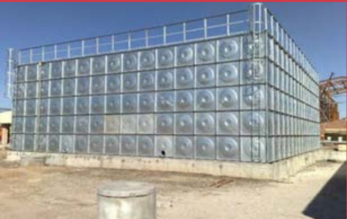
Fire Water Storage Tank
