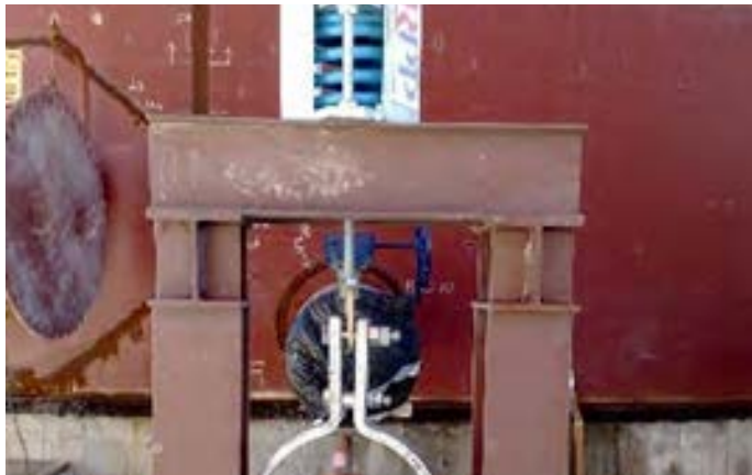
Piping Spring Hanger Support
