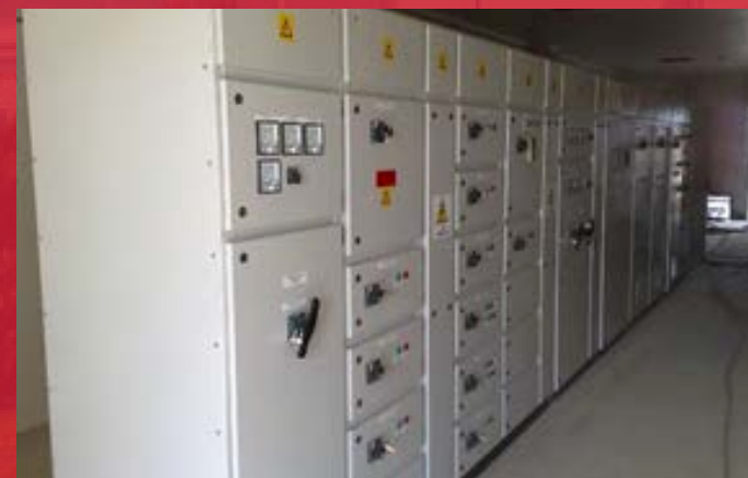
MCC Cabinets Ready for Handover
