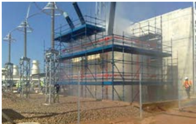
Transformer Fire Water Spray Test
