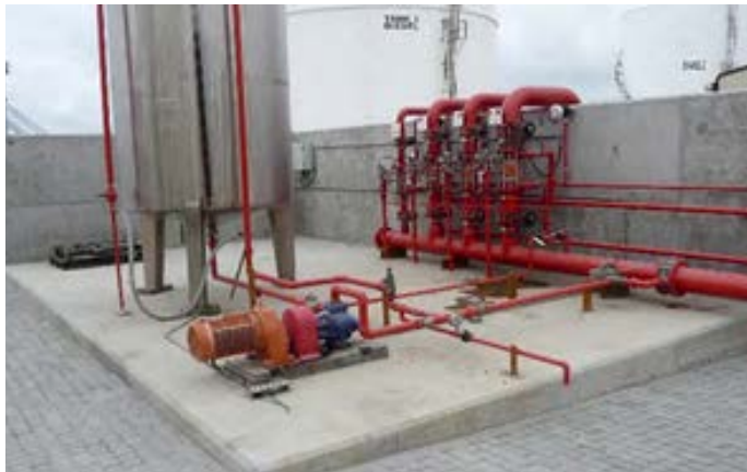
Bund Area Fire Foam System
