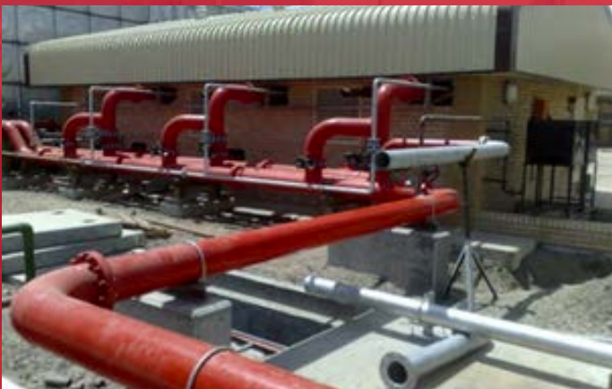
Fire Pump House and Piping
