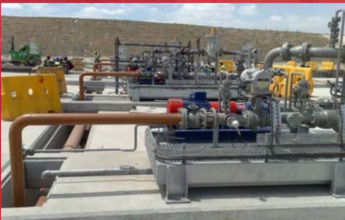
Gas1 Diesel Truck Off-Loading Stations
