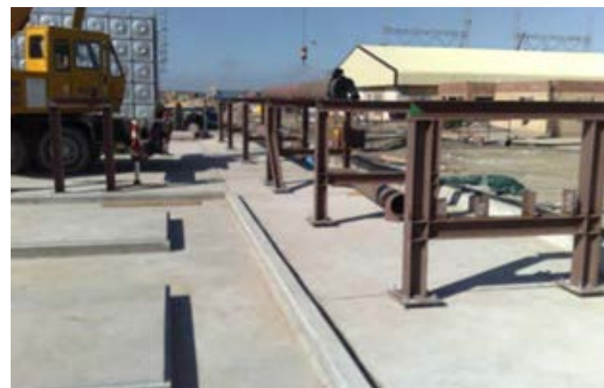
Overland Pipe Supports
