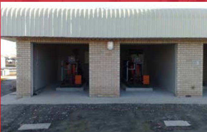
Fire Pump House
