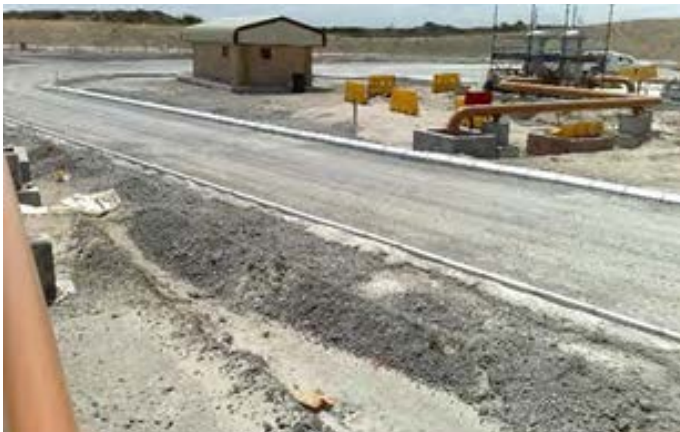
Fuel Pipeline Road Crossing
