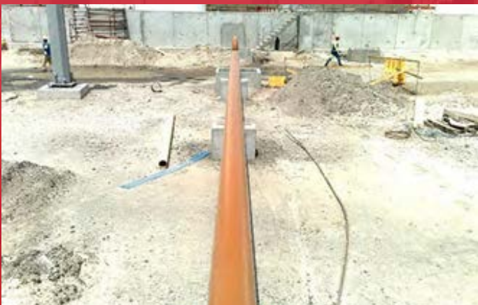
Overland Fuel Pipeline
