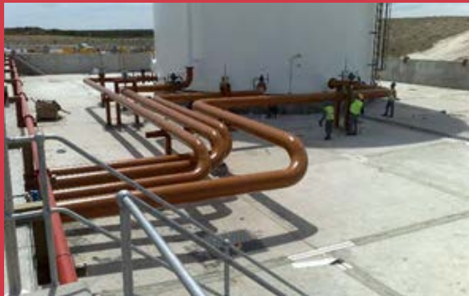
Fuel Piping Ready for Hand Over
