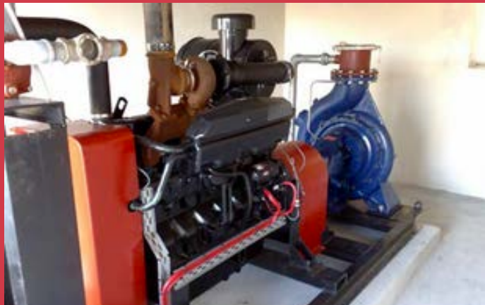
Diesel Fire Water Pump
