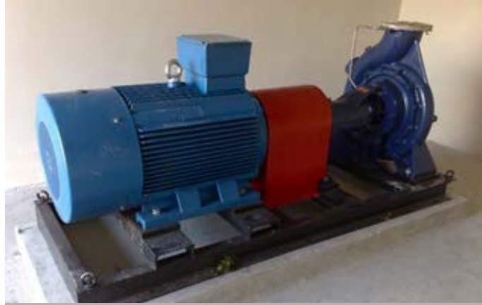
Electric Fire Water Pump
