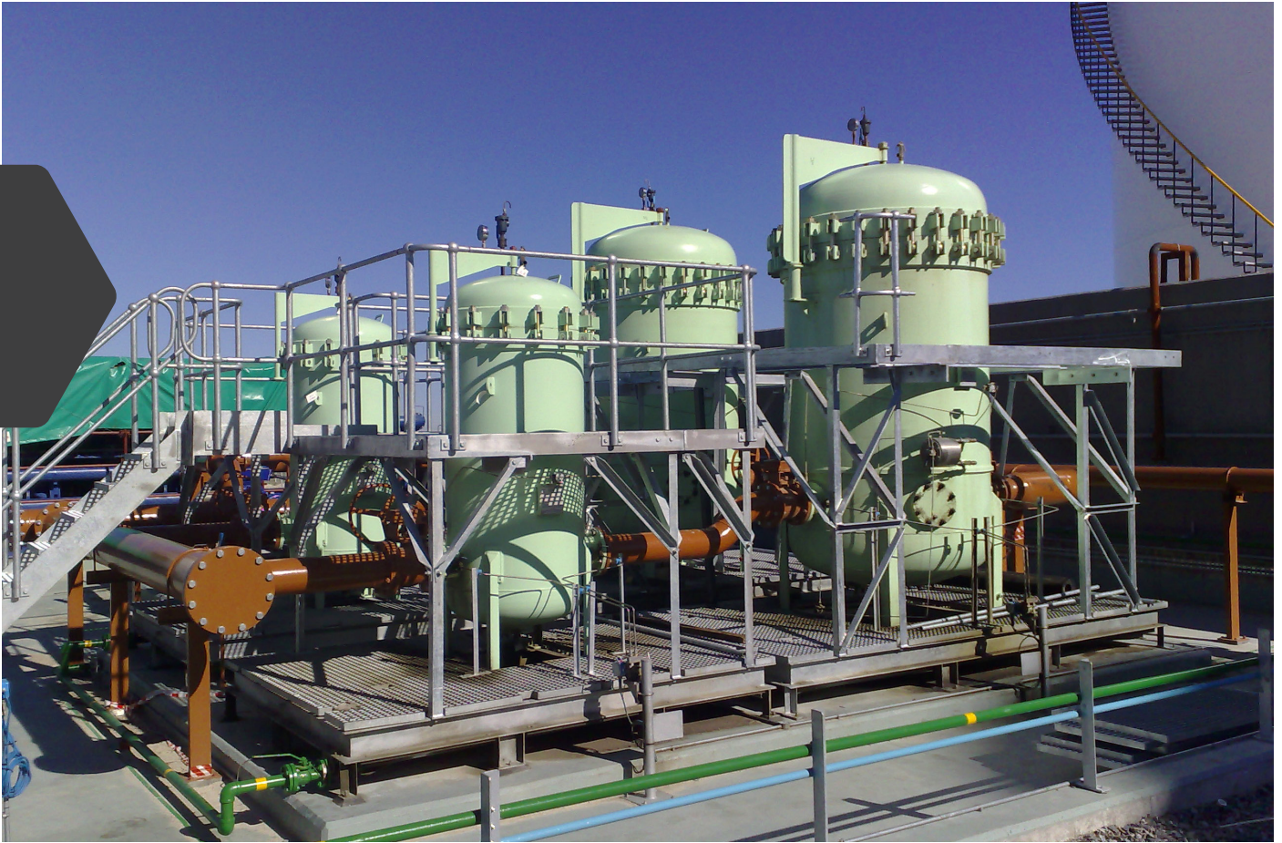
OCGT Atlantis Fuel Filters
