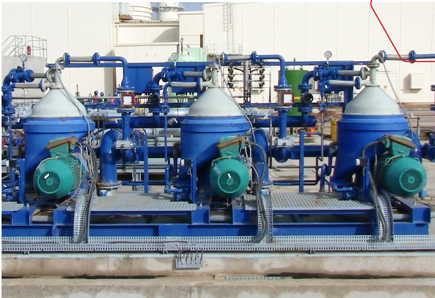
OCGT Mossel Bay Fuel Treatment Plant 1
