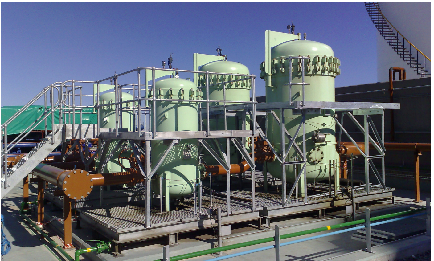
OCGT Atlantis Fuel Filters
